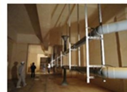
2,000 t Heat storage tank (Underground Pit)
