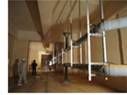
2,000 t Heat storage tank (Underground Pit)
